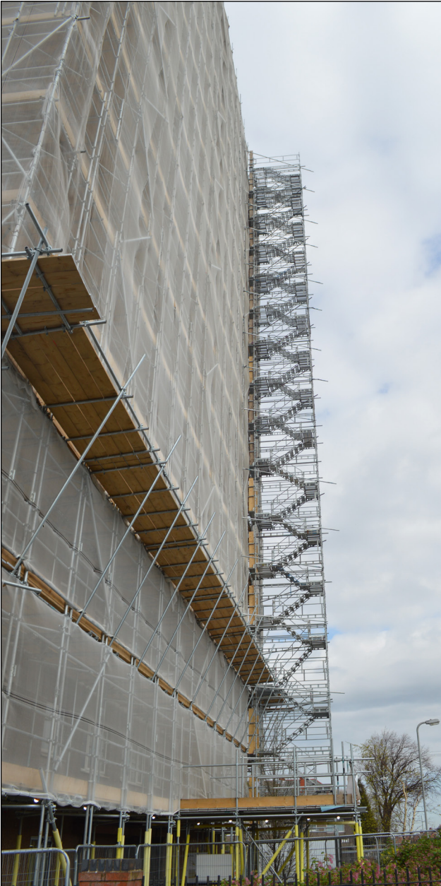
Figure 7 Where sheeted scaffolds form part of the escape route, do not sheet the stairways or ladder points so that smoke can escape and the fire and rescue service can gain access
