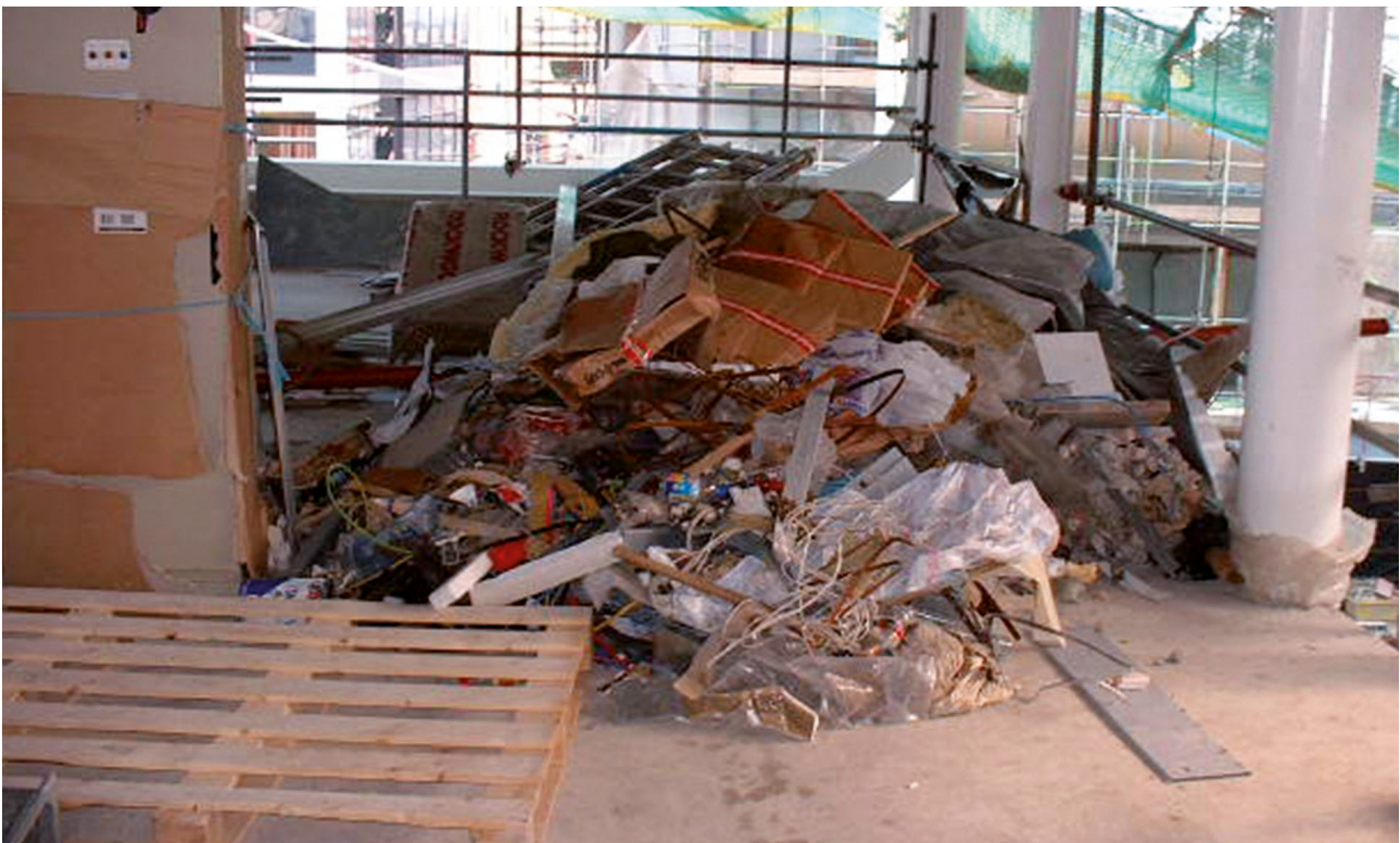
Figure 8 Most construction rubbish can burn. Make sure that it is cleared up and removed from the site as soon as possible
