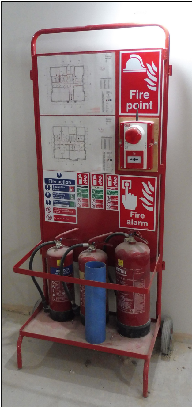
Figure 16 An example of an interconnected alarm and fire extinguisher point in a refurbishment project. Most sites will require an interconnected alarm system (either wired or wireless)
