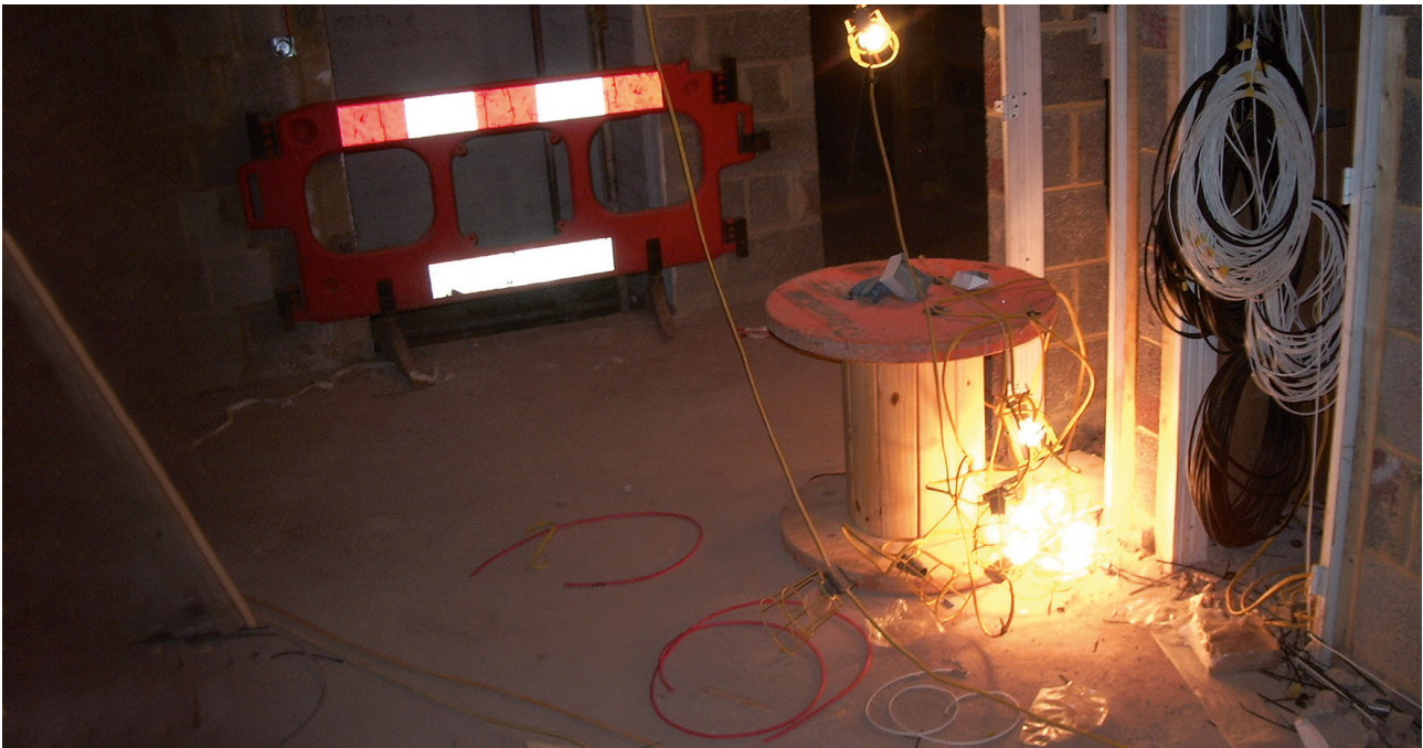
Figure 4 Festoon lighting: poor positioning creates a potential fire risk
