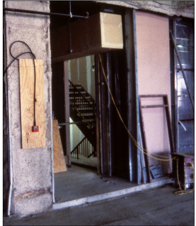
Figure 13b This escape route will quickly fill with smoke in a fire because no fire door is fitted
