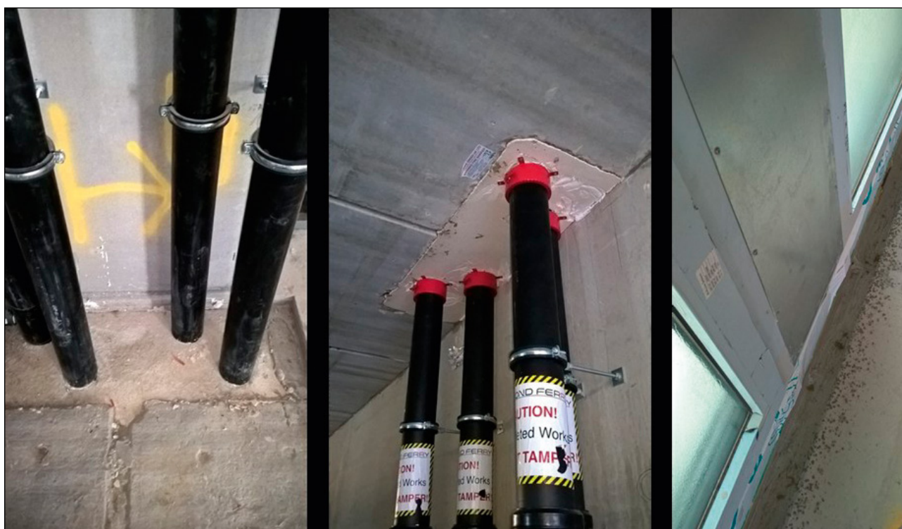
Figure 15 Fire stopping installed around penetrations made for services and in the gap around windows
